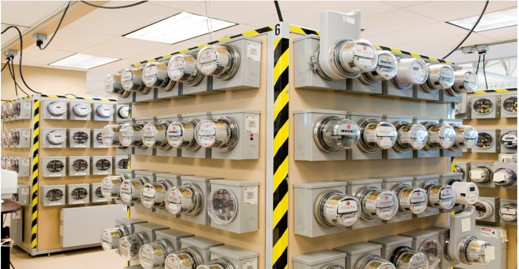
Typical Metering Farm
